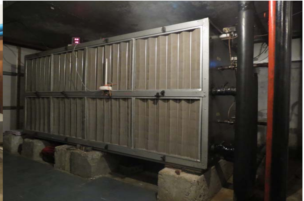
AHU room with cooling coil
